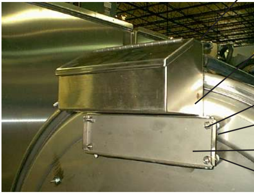
flow restrictors installed here
